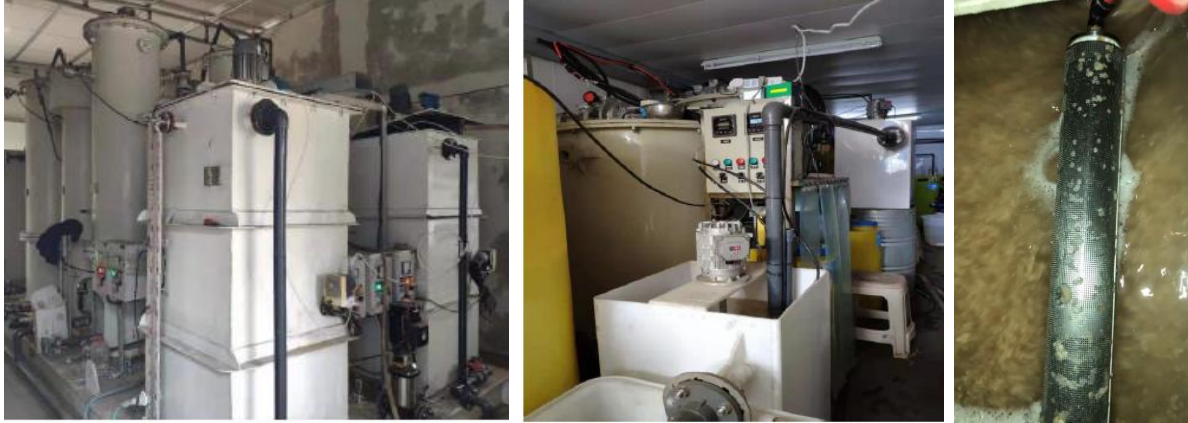
Figure 3. Photo of the Pilot Plant Equipment, CIF® (left), BIOCLENS® Reactors (middle), Self-Cleaning Screen (right)
