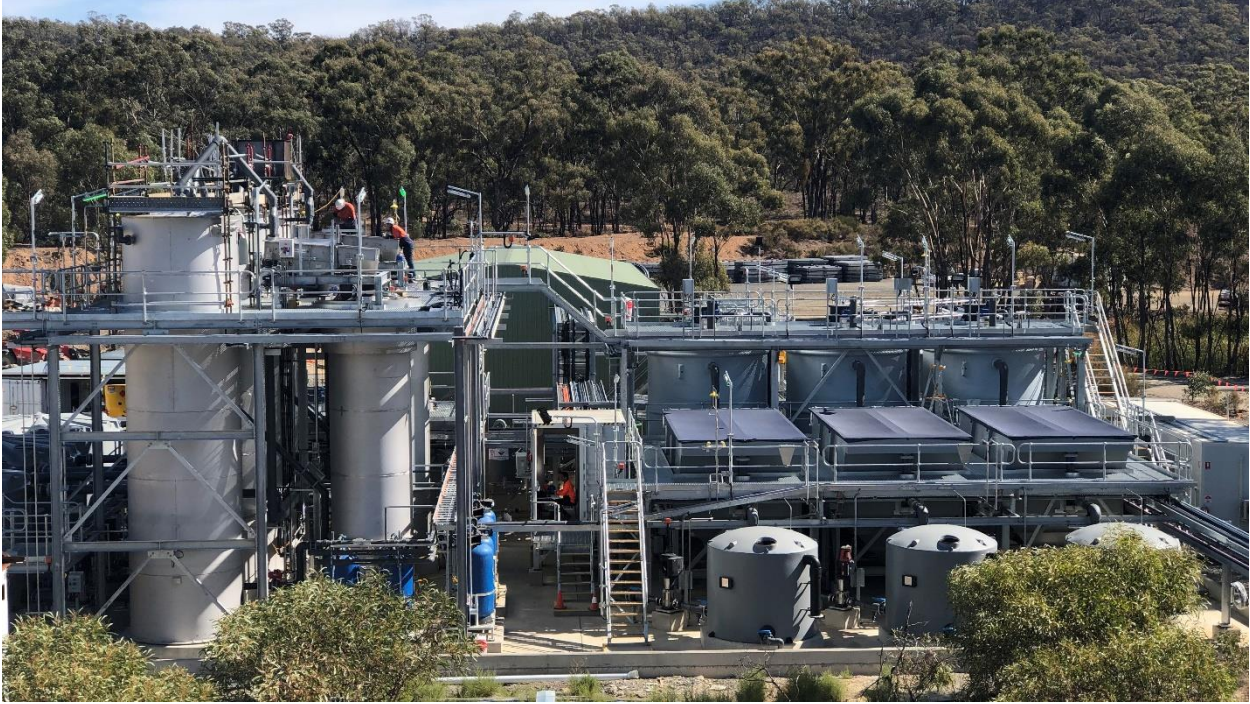
Figure 3. Photo of the Completed Plant
