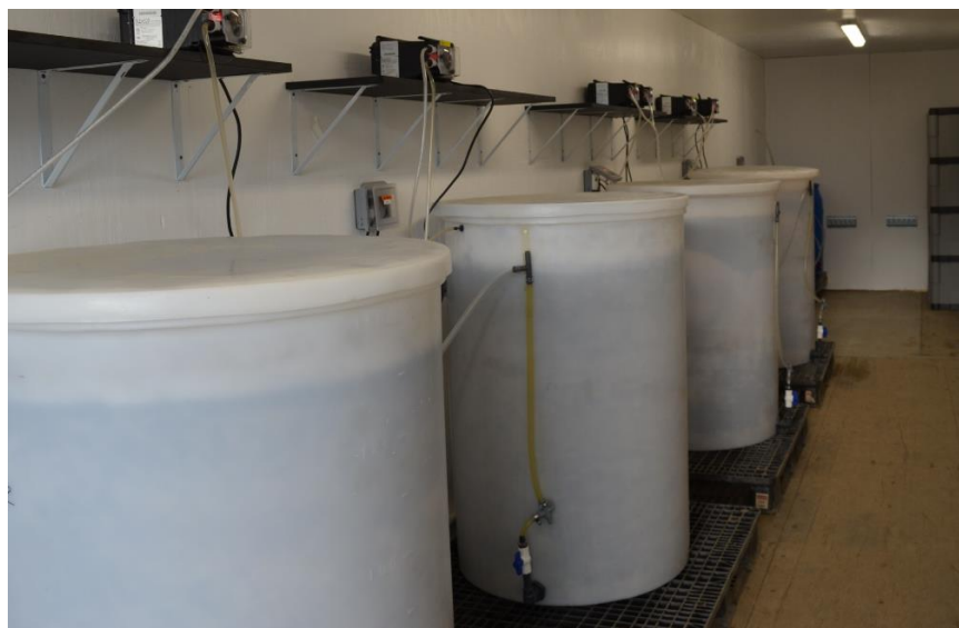
Figure 4: Primary treatment sulfate reducing bioreactors
